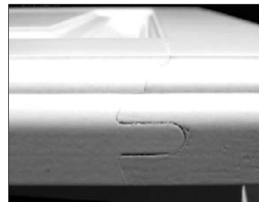
Example of end joint separation
