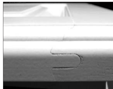
Example of end joint separation
