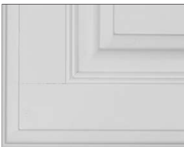
Example of front joint separation
