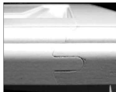
Example of end joint separation
