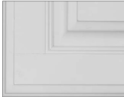
Example of door front joint separation
