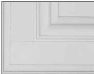
Example of front joint separation
