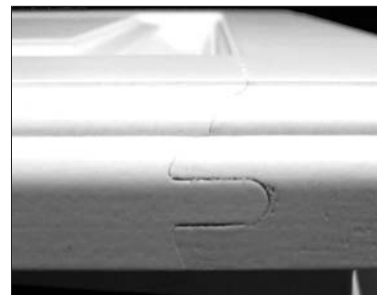
Example of end joint separation
